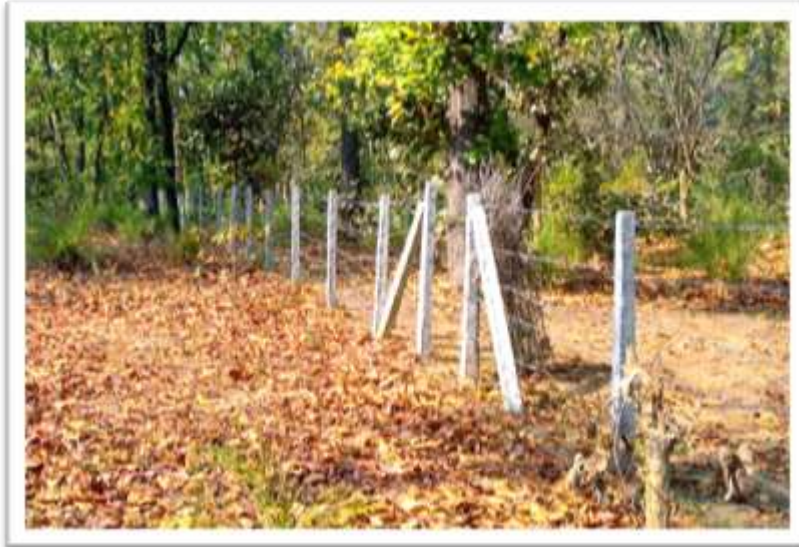
View of Barbed wire fencing completed in Preservation plot Shahdol (Lamer) forest division
